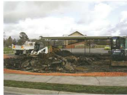
Work has officially begun on the Main Oval Pavilion with site preparation works commenced on Thursday July 12, 2007
